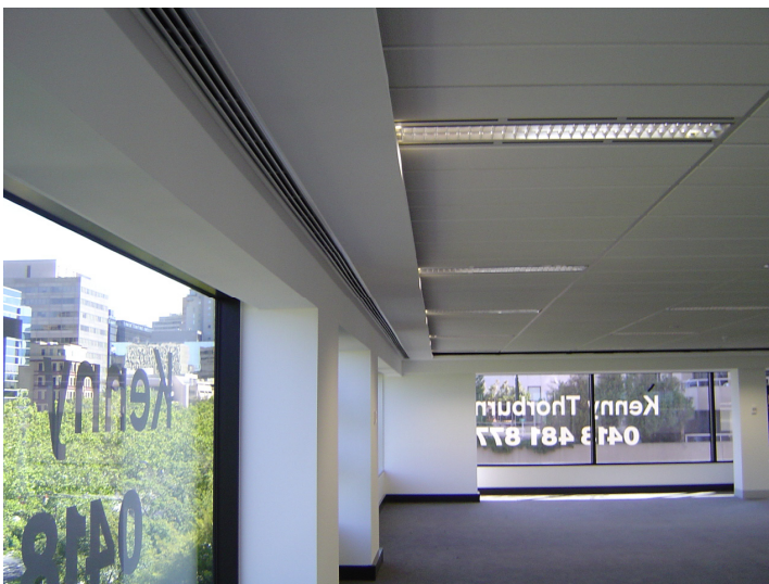
Continuous Linear Perimeter Grille and Ceiling Mounted Terminal Units
