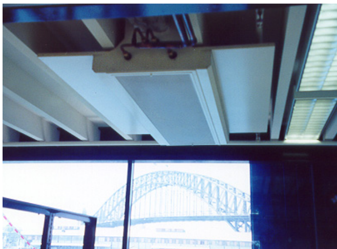
View of Active Chilled Beam installed between ceiling joists
