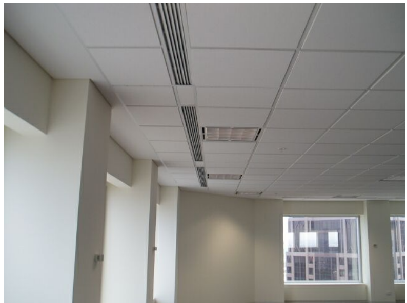
CM10 Units with 'Lay-In' Supply Air Grilles
