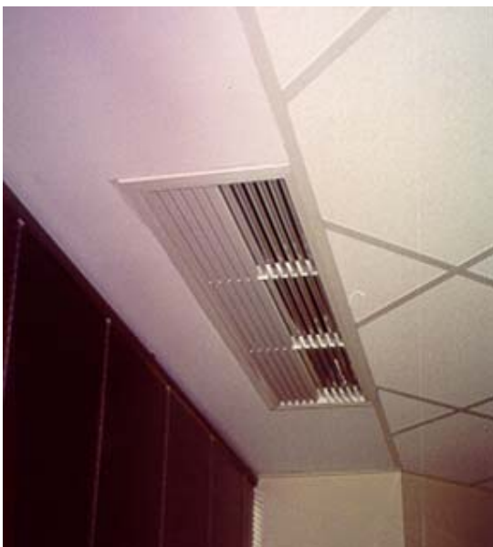
CM10 Units with Combined Supply/Return Grille in Plaster Ceiling Margin
